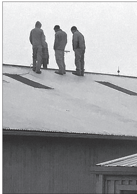
Minna Construction replaced the tornado damaged roof of the Riding Centre's indoor aren in late December, braving Ohio winter and working with the needs of both riders and horses PHOTO: CAROLYN BAILEY
